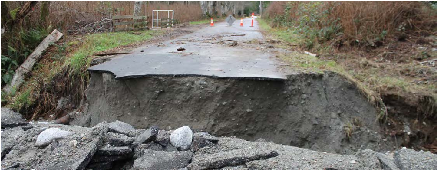
Russel Road washed away from heavy rain, Sunshine Coast, Donna McMahon
